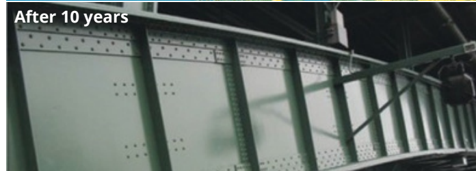
Peace Bridge The Peace Bridge, connecting Buffalo, New York and Canada, was coated with PSX 700 more than two decades ago. Despite brutal winter and humid summer conditions, the bridge has retained the gloss and color of the initial application.
