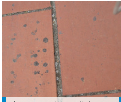
An example of old terracotta floor requiring treatment before applying Aquaflex Roof
