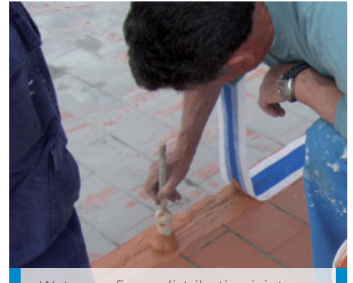
Waterproofing a distribution joint with Mapeband fixed in place with Aquaflex Roof
