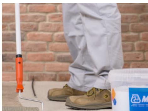
Application of Primer 3296 as substrate preparation in the reinforcement of brick concrete slabs with Planitop HPC Floor
