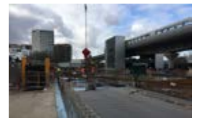
Proofex Engage installed
